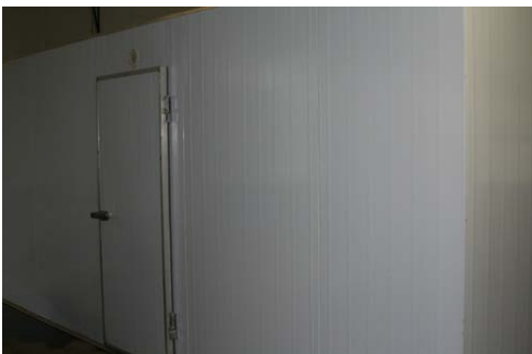
Walk-in cold room and freezer
